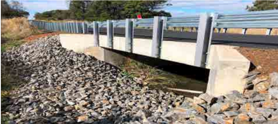
Kadnook Connewirricoo Road Bridge over Kadnook Creek – new deck overlay and guard rail
