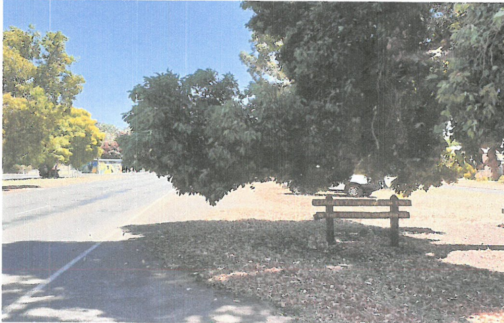
Large limb intruding onto the Wimmera Hwy.
