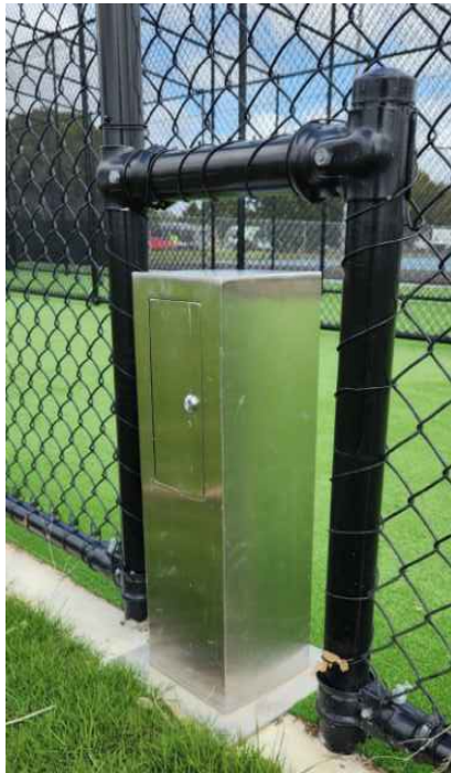
TYPICAL POWER BOLLARD INSTALLED WITHIN NEW FENCE LINE.
