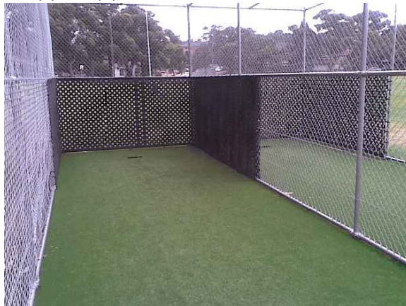
TYPICAL RUBBER BELTING - TO BE INSTALLED ALONG THE NORTH AND SOUTHERN SIDE OF FENCE - 61m
